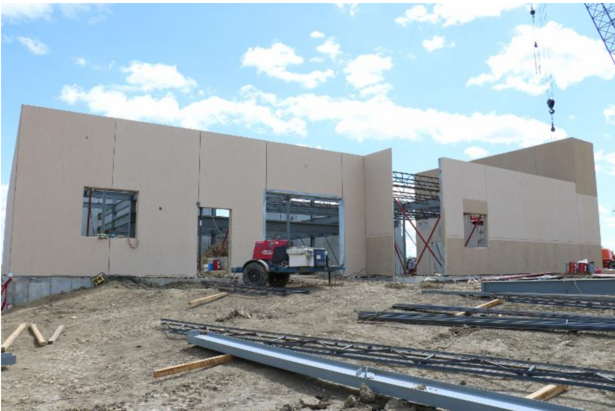
Looking up and toward the east, this is the facilities/utilities area on the left and the kitchen area on the right. These are the first pre-cast walls that were placed on the campus.
