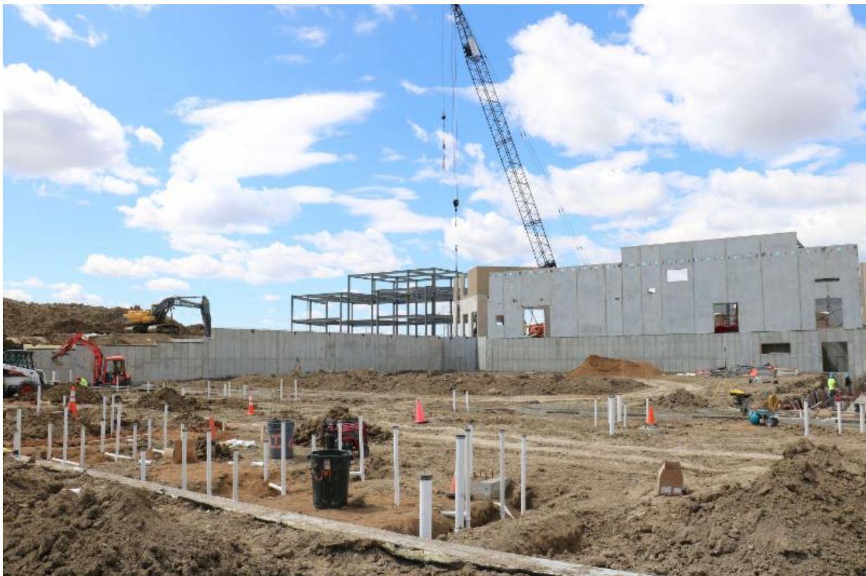
This photo is facing west, looking at where the locker rooms and gyms will be located. The steel structure in the background left side is the Academic Center.
