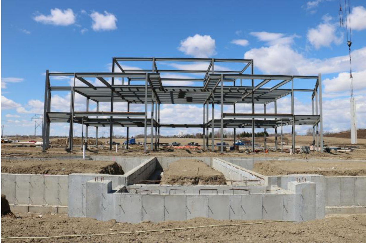
Looking to the west, this is the view of the new SMCHS Academic Center. The first pieces of structural steel were placed in this area of the campus. This is the courtyard view of the future main entrance.
