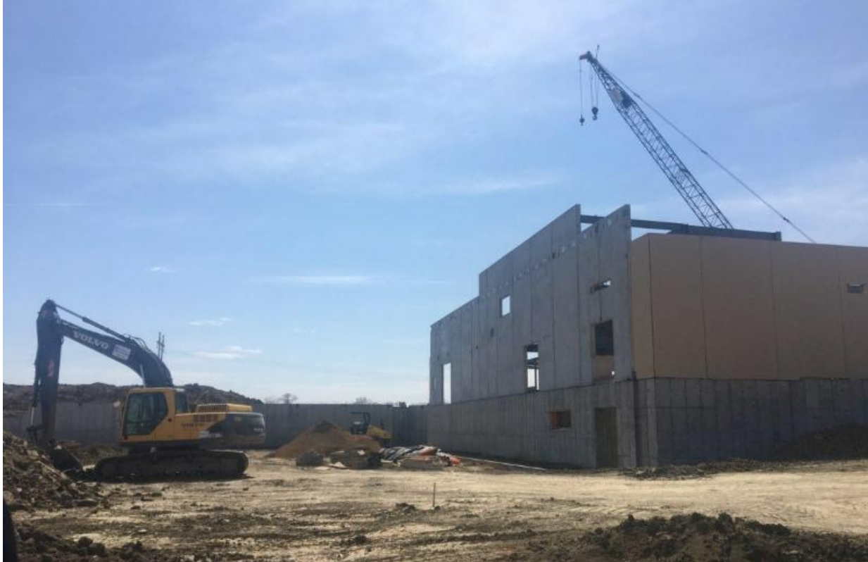
In the Athletic Center area, the top-loading gym area is visible on the left side of this photo, and the facilities/utilities area is on the right.
